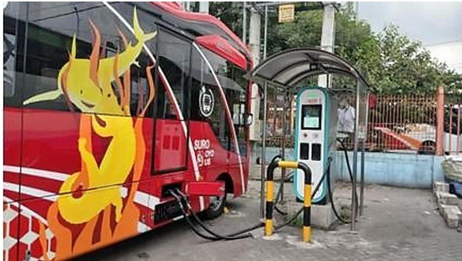
Figure 10. Suroboyo Electric Bus charging process
