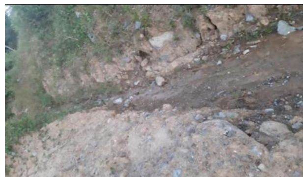
Figure 3. Documentation The boundary of the excavation depth from the initial soil surface
