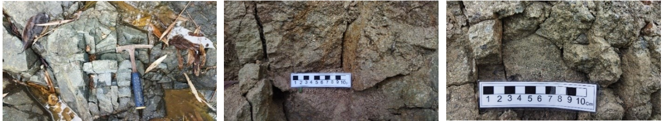
Figure 11. Joints appearance (from left to right) at Loc 41, 50, and 95.
